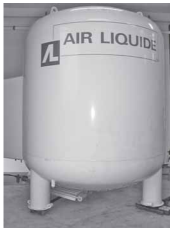
Nitrogen tank for the cooling system
